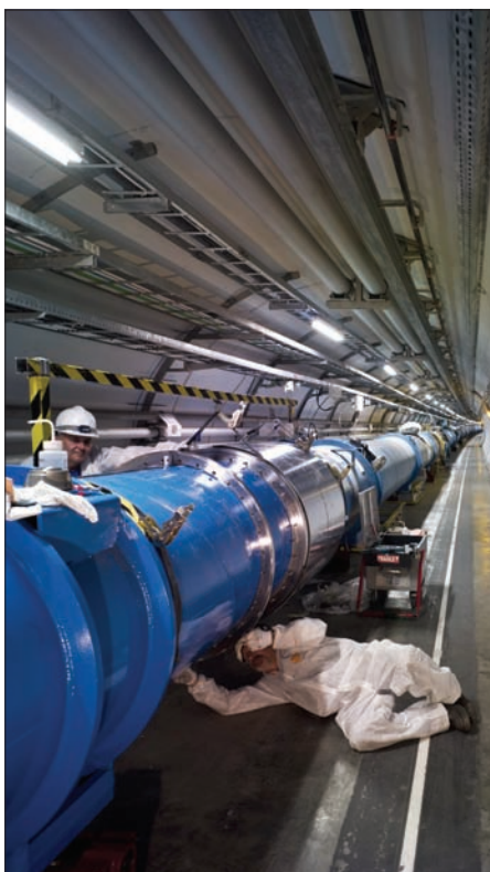
A magnet interconnection being closed in Sector 5-6 at the end of June, following repairs to the copper stabilizers. Tests completed for all sectors show that the machine is safe to run in 2009–2010.
